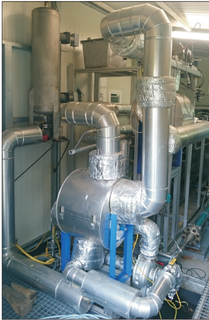
FIG. 3. CORC setup in a container that was placed outside of the laboratory due to safety reasons. Heat exchangers and piping system were thermally insulated with mineral wool.
